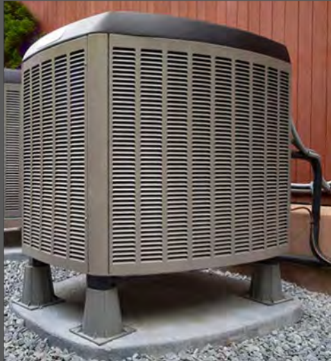
Heat Pump Space Heating/AC
